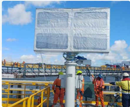
BAS Installation at Dolphin
