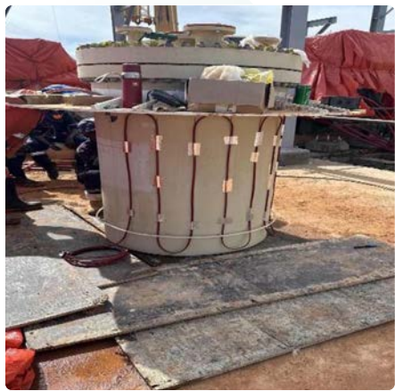
Electrical Heat Tracing (EHT) on Seal Oil Drum
