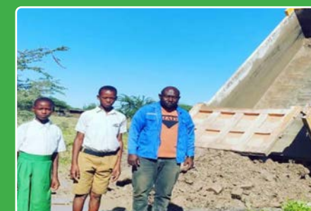
Dumping the unused concrete on the community/ school access road
