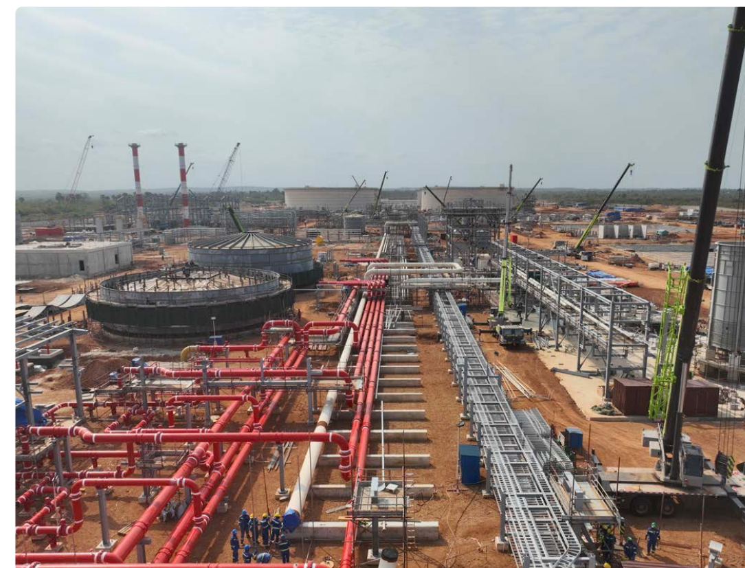
Along Tank C Pipe Sleeper (From Jetty To Tank)
