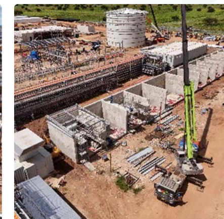
Electrical, Instrumentation, Telecommunication and Security Systems (EITS) Transformer Shelter Installation
