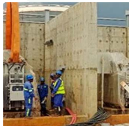
Distribution Transformer Installation
