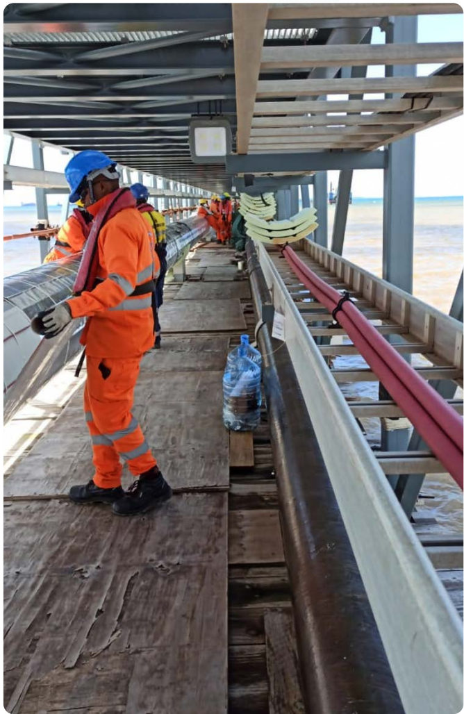
Oil Export Electrical Heat Tracing (EHT) & Insulation
