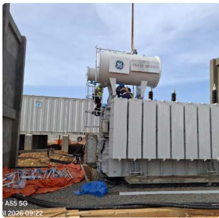
40MVA Shunt Reactor Assembly
