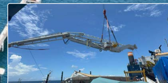
Three Marine Loading Arms (MLAs) Installed
