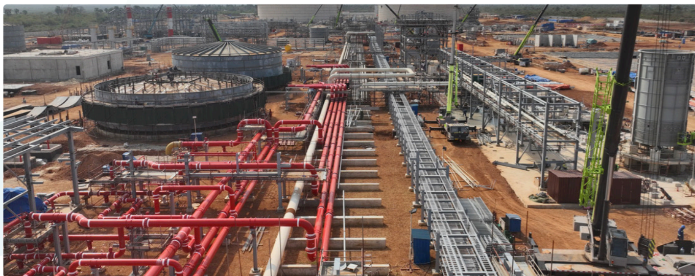
Along C1 Pipe Sleeper (From Jetty To Tank)
