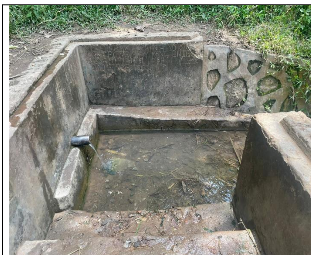
Protected spring well in PPL RoW, Kijumba Village, Hoima District
